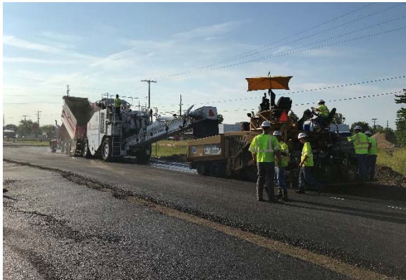
One of our paving crews laying down the layer of asphalt that allows the road to drain. This layer is known as open grades.
