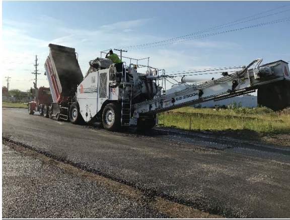
Asphalt being dumped into our shuttle buggy which loads the paver with asphalt
